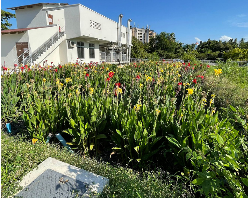
Gravel Filtration for Wastewater at CCBRT Hospital in Dar es Salaam, Tanzania. © Avantika Singh, UNEP.
